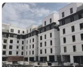
DARCO Signature Jeddah, Saudi Arabia | Apartment
